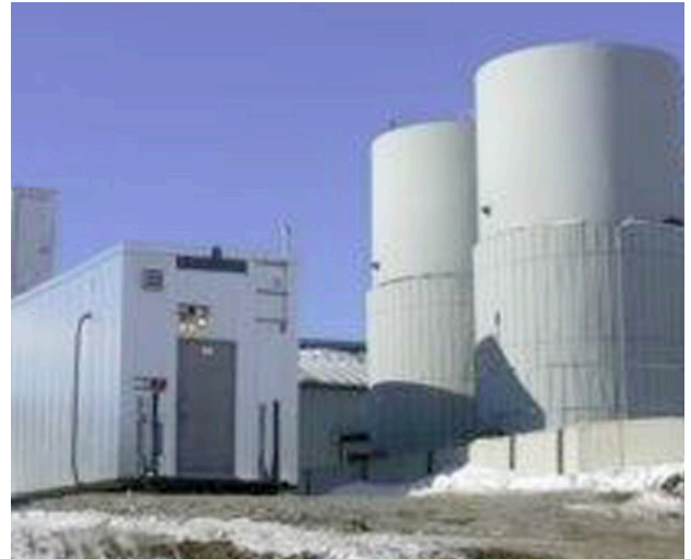
Water storage tanks and Total Fluid's treatment skid near Drayton Valley
